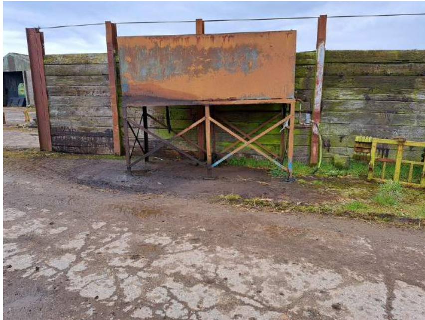
Image 8.6 Unbunded, above-ground fuel tank with minor spillage
